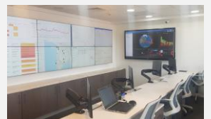
NOC, IoT platform, Remote Management and Monitoring Centre
